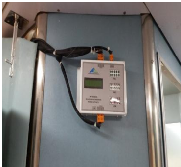
Fig.10: Water level indicator (Display) (Inside of coach)
